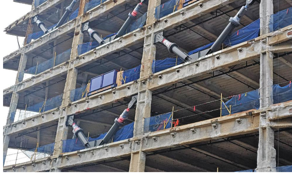
Figure 1 Example of a distributed damper configuration along the perimeter of a steel building.
