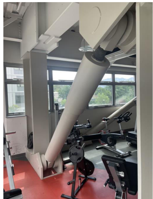
Figure 5. Dampers with integral extenders within SidePlate® moment frames at the Salt Lake City Public Safety House
