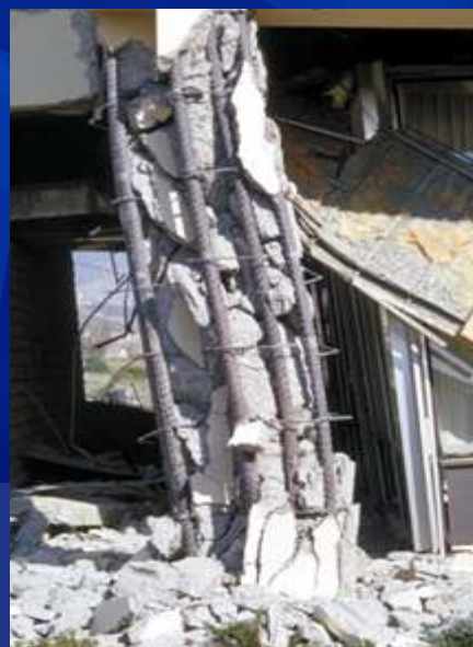
Olive View Hospital – failed tied column. (Source: NISEE-PEER, University of California, Berkeley)
